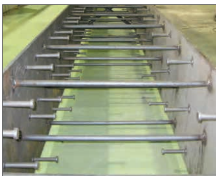
▽ Steel-concrete-steel test specimen prior to concreting (carbon steel plate on the left, stainless steel plate on the right)
